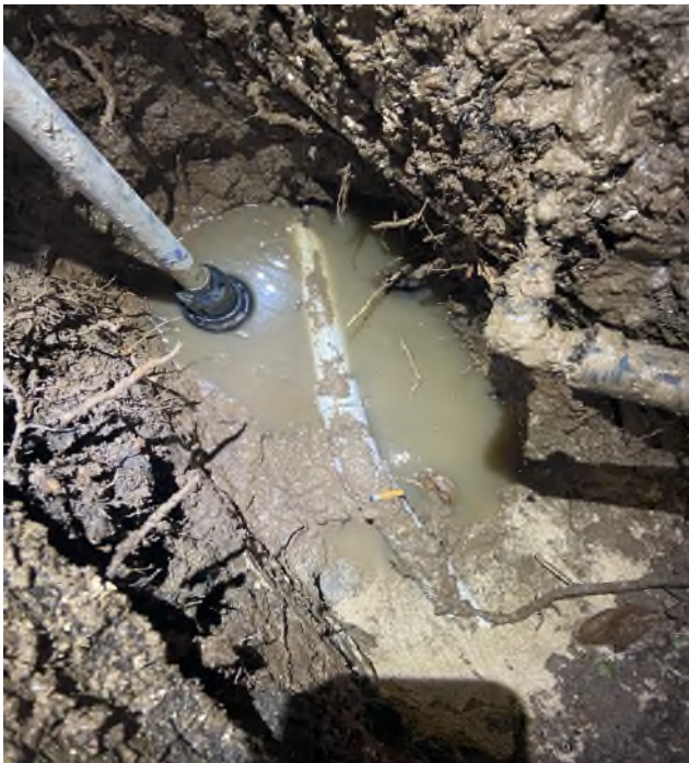
3. Found that roots damaged the piping.
