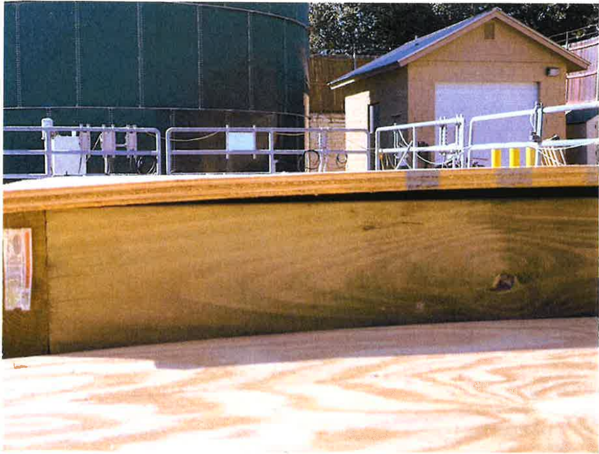
Figure 4: Large Gap at Removable Equipment Access Cover
