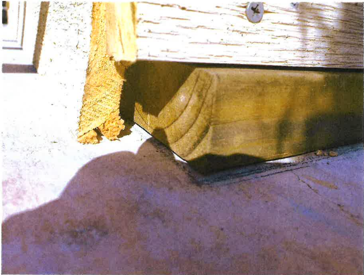
Figure 2: Gap at the interface between the fascia and the joist
