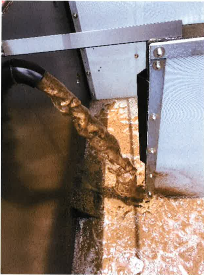
View inside sludge box during automatic wasting.
